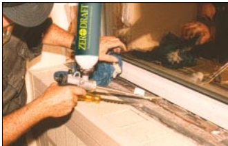
Zerodraft Foam Sealant being applied to seal gap between window frame and rough opening.
